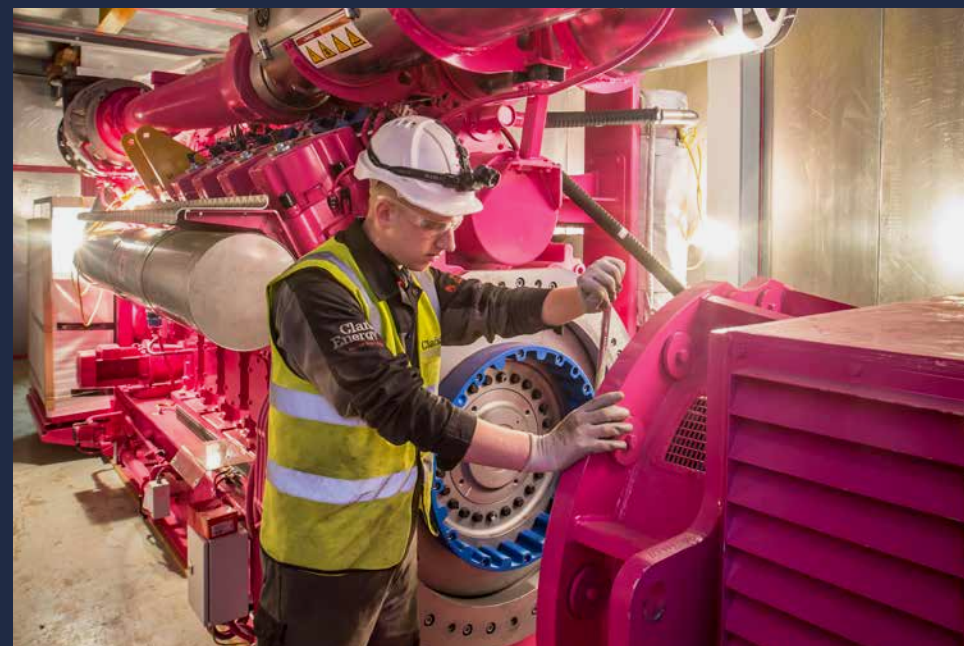
Biogas powered CHP engines in our energy centre.
